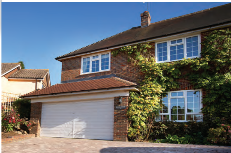
A two-storey extension incorporating an integral double garage and extra bedroom above.
